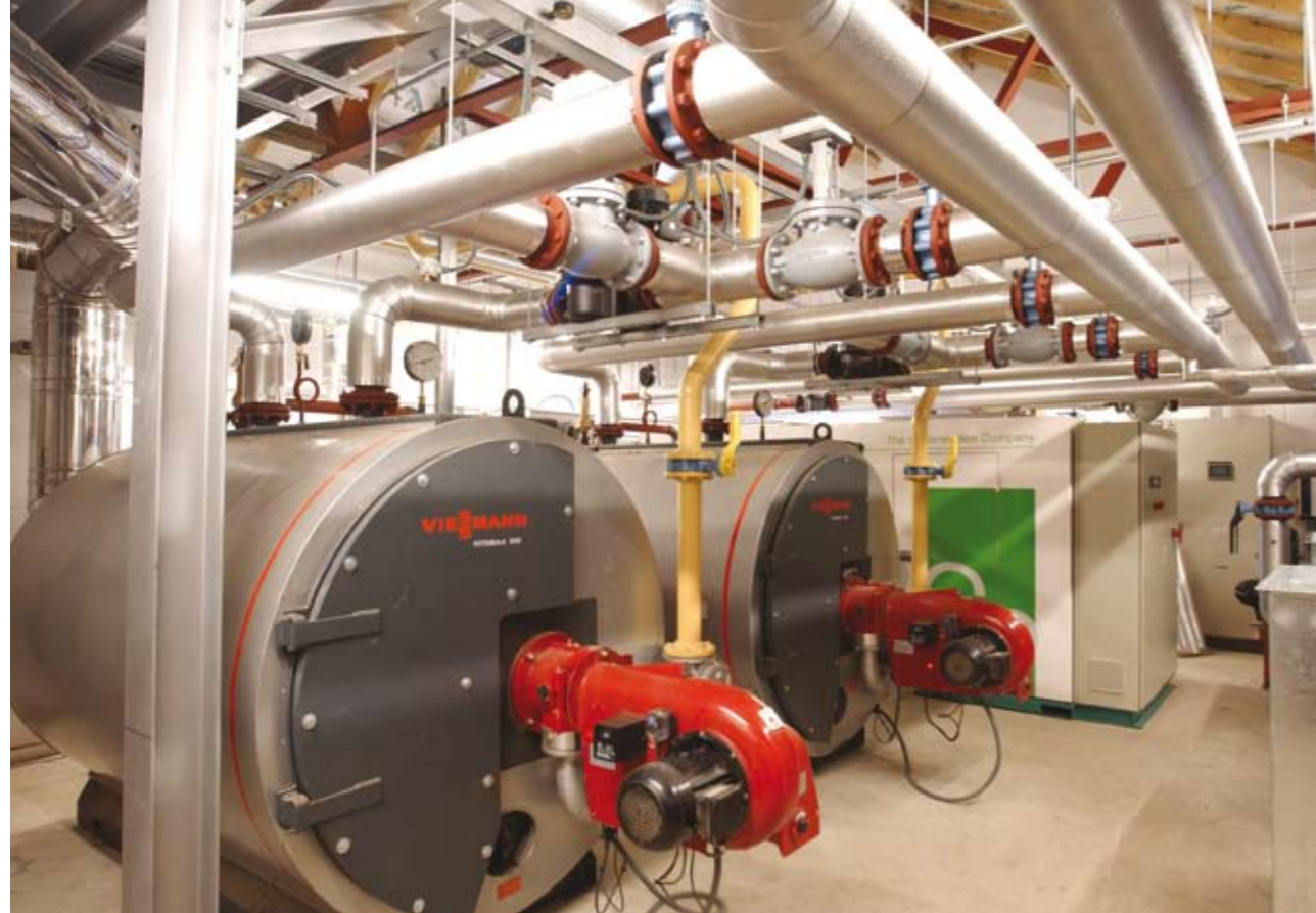
Figure 8: This shows the interior of the Stockethill plant room, Aberdeen
